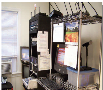
Kennebunkport Control Room
